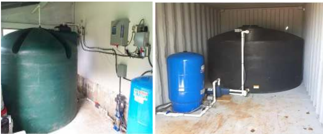
Figure 1.2: Water storage tanks
