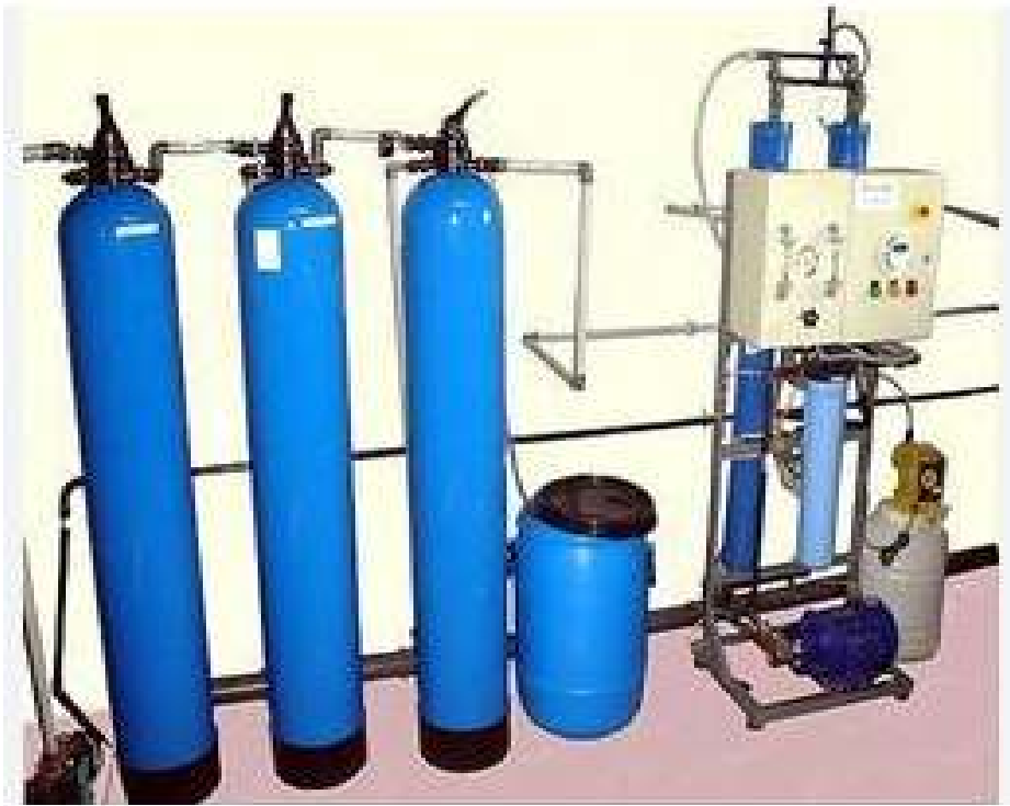
Figure 1.10: Reverse osmosis plants
