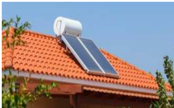
Figure 2. 4 Solar water heater
