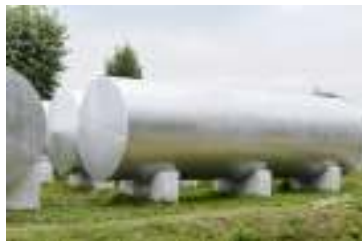
Figure 3.1 Aboveground storage tanks
