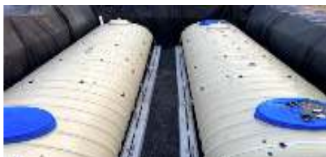
Figure 3.2 Underground storage tanks
